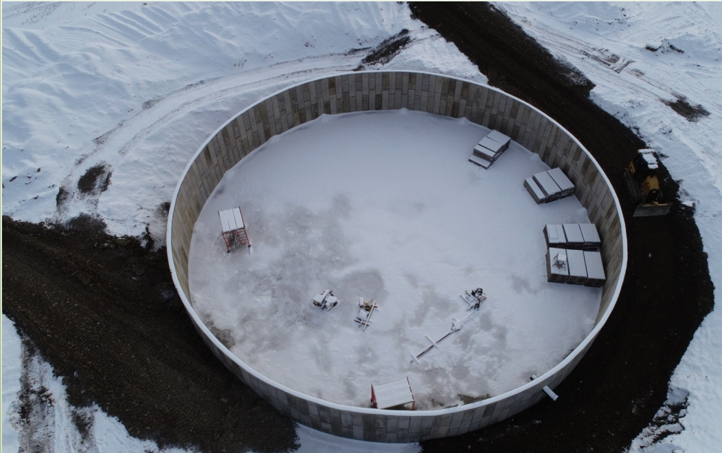
Manure storage project during construction this winter funded with NYS Agricultural Nonpoint Source Pollution Abatement & Control Grant and USDA Environmental Quality Incentives Program.
